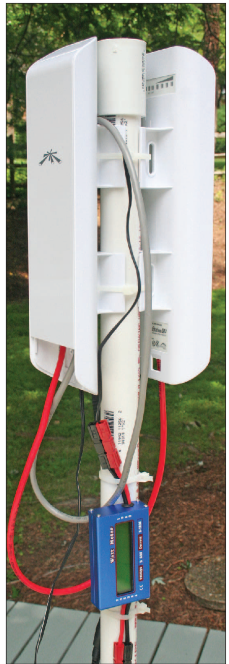
Figure 6 — Two back-to-back NanoStation M3 stations connected by an Ethernet cable function as a wireless network relay station. The blue box at the bottom monitors voltage and current.
